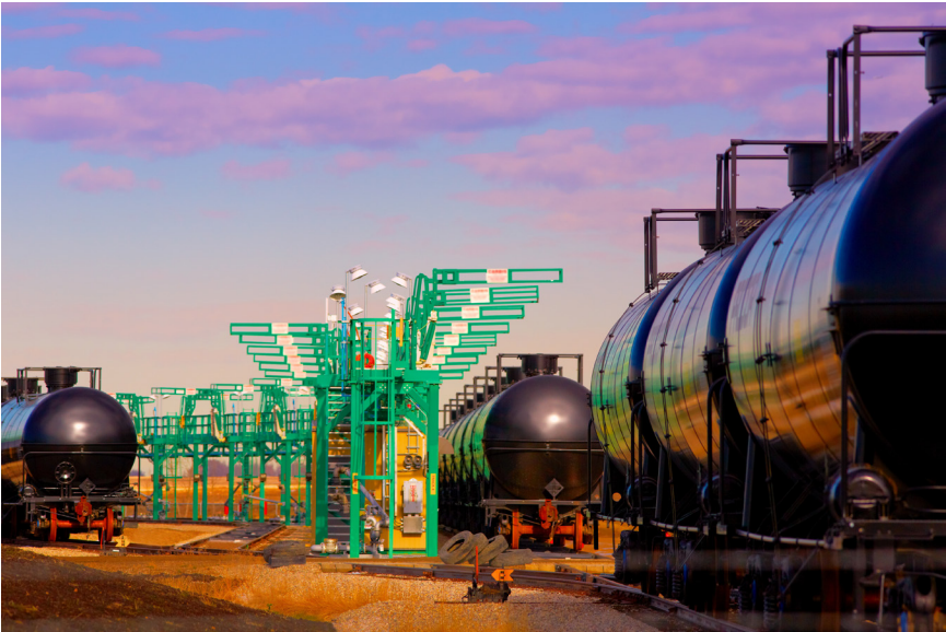
FIGURE 3-12 Siding loop (a) and crude oil-loading rack (b) for unit train service.
