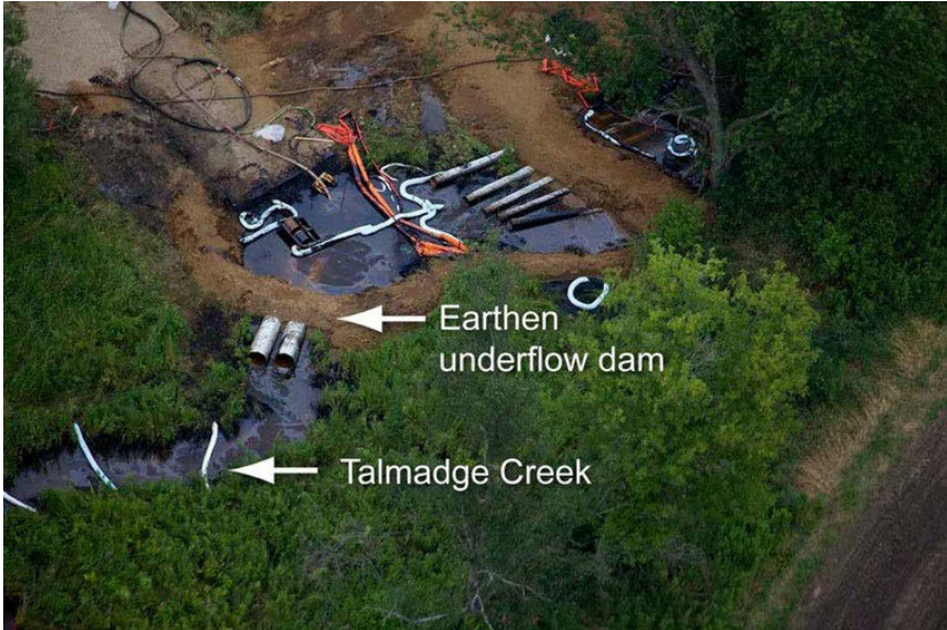
FIGURE 4-11 Efforts undertaken to contain and collect the release of heavy crude oil from the July 25, 2010, rupture of a hazardous liquid pipeline in Marshall, Michigan. Picture of site was taken on July 30, 2010.
